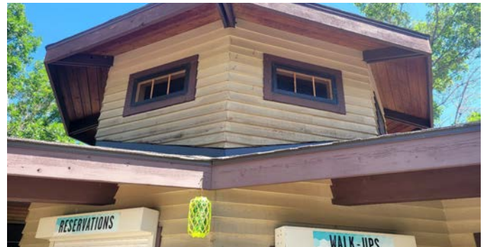
Existing Concessionaires Building Exterior Deterioration
